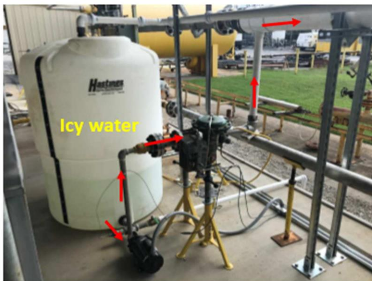
Figure A.9 Cooling System
