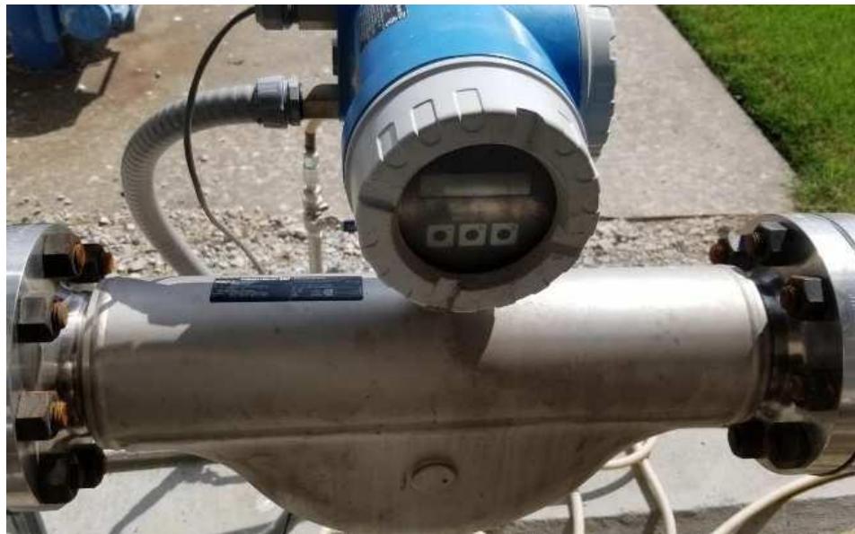
Figure A.3 Coriolis Flow Meter
