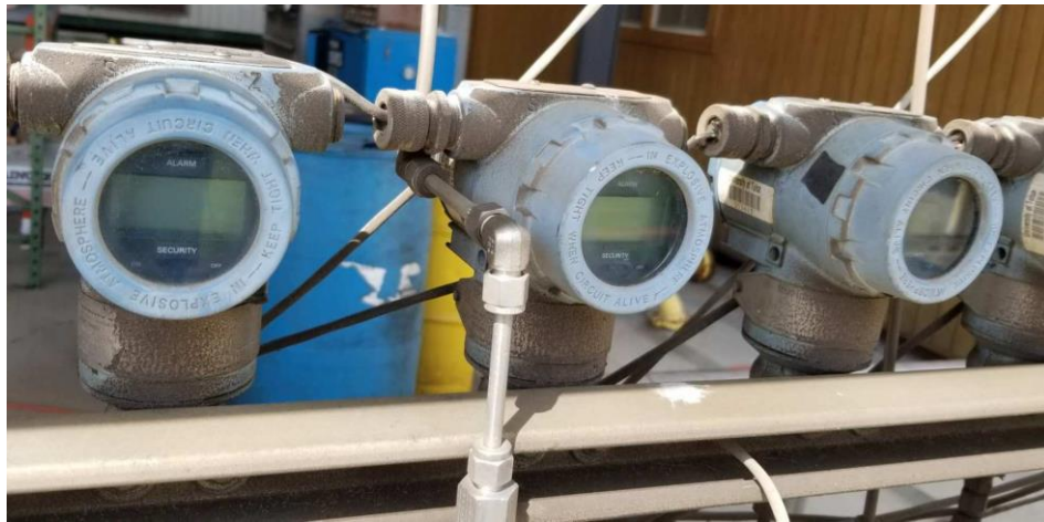
Figure A.7 Pressure Monitors
