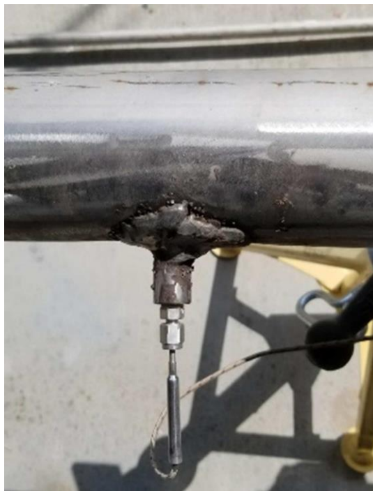
Figure A.5 Temperature Sensor
