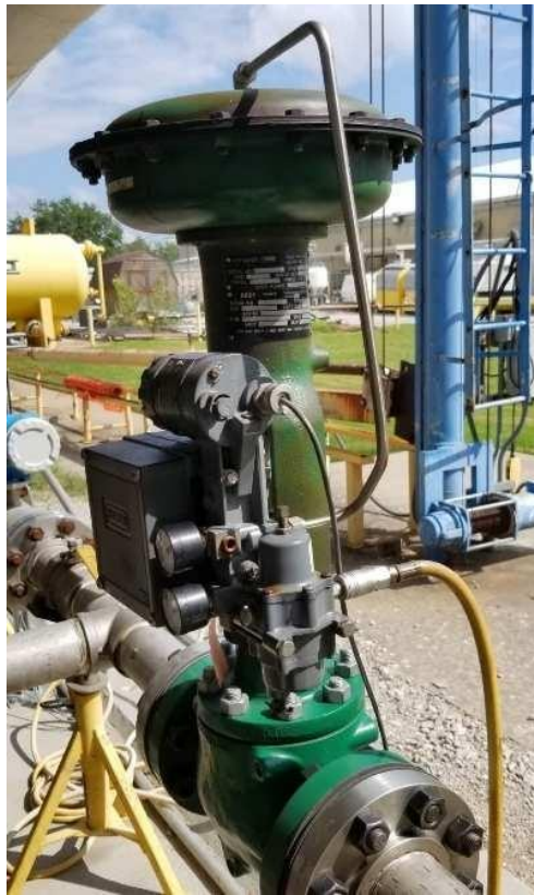
Figure A.8 Pneumatic Control Valve
