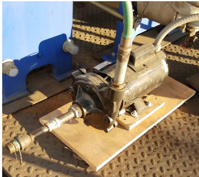
Figure A.6 Heat exchanger pump
