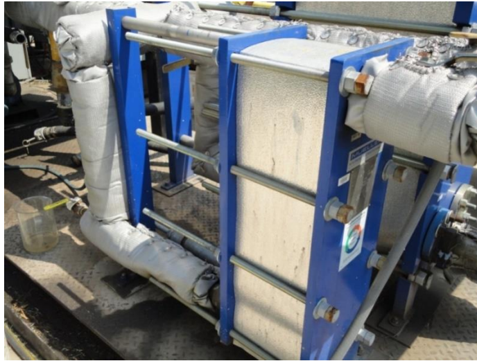
Figure A.5 Heat exchanger
